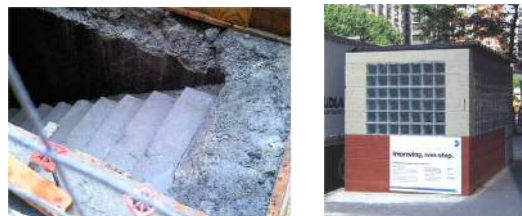
Recently uncovered stairway originally constructed in the 1980s and the structure now in place atop it to allow access by workmen and their equipment.
