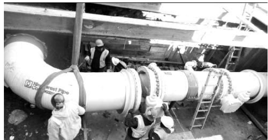
Workers installing a 48-inch double butterfly valve in its chamber on E. 59th St. between 1st Ave. and 2nd Ave. Butterfly valves isolate sections of the trunk water main for maintenance purposes.
